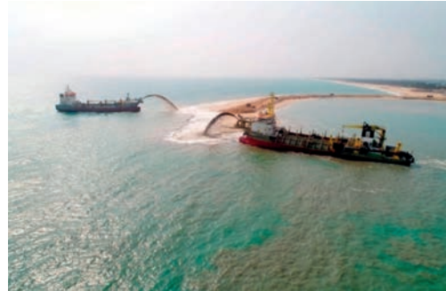
Figure 2: Trailer Suction Hopper Dredger rainbowing sand to create the Sandbar Breakwater (Source: Boskalis).
