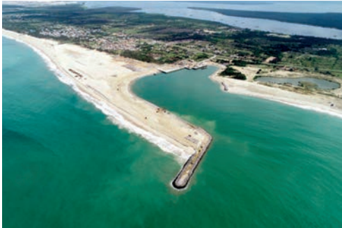
Figure 1: Aerial view of the Dangote Project. The Sandbar Breakwater is under construction. Only the outer tip is protected by armour rock (Source: Boskalis).
